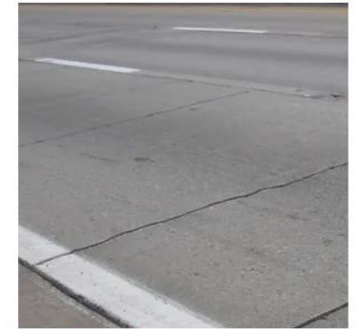
Low-Severity Transverse Cracks
