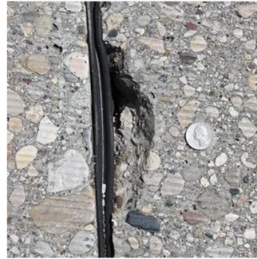
Spalled Joints and Cracks
