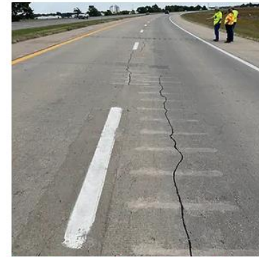
Low-Severity Longitudinal Cracks or Joints
