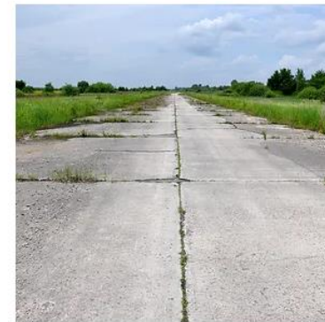
Joint Sealant Failure
