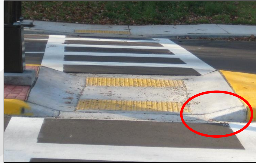
Undesirable – sloped edge
